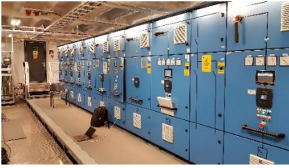
Power measurements on board
