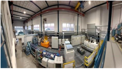
The physical Zero Emission Lab, containing a fuel cell, hydrogen, a modern dual fuel generator set, and sophisticated electrical power distribution.
